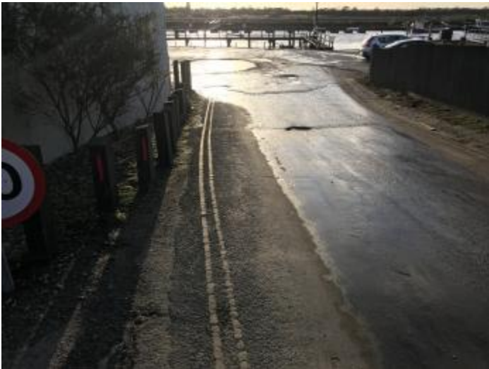
Drop Off For Rear Entrances
